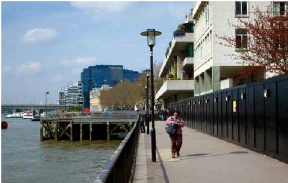
Sugar Quay building prior to demolition with existing jetty - From the East
