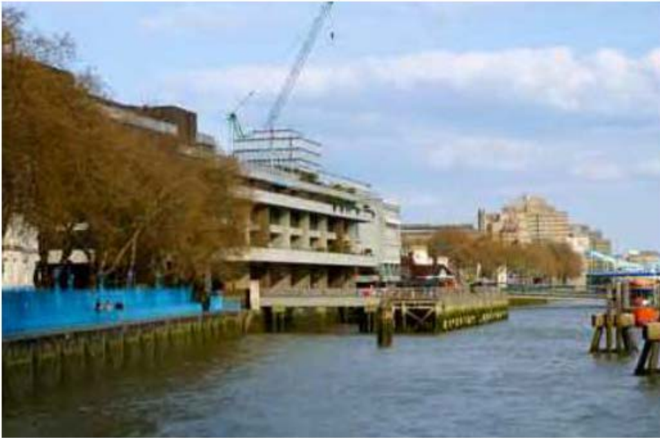
Sugar Quay building prior to demolition with existing jetty - From the West
